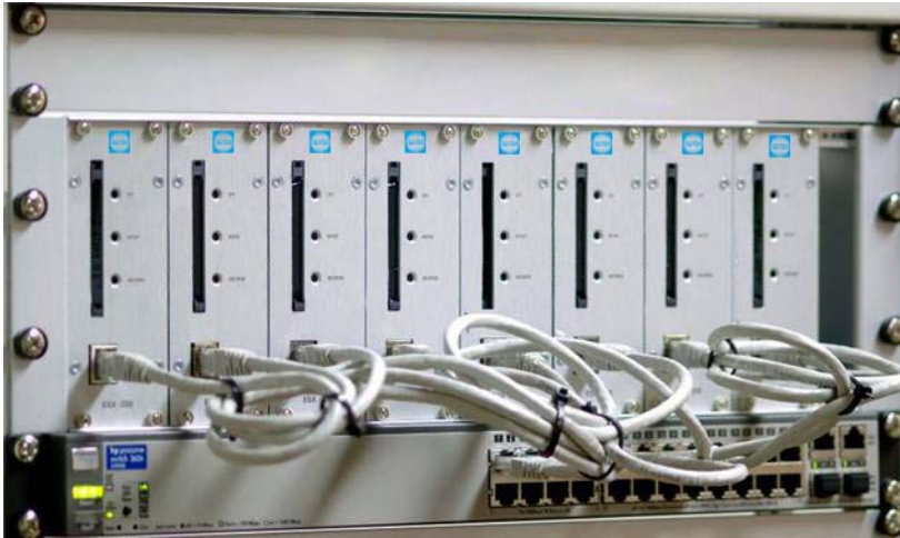
OTX 0200 connected through a switch with DHCP
